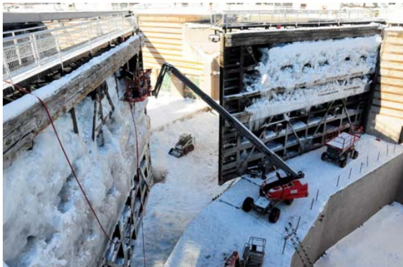
Deicing gate to allow maintenance to be performed during winter work
